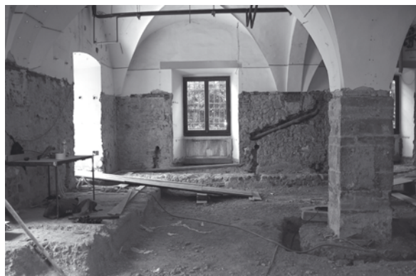
Conversion of the former printshop into storage area for more than 70 000 volumes
